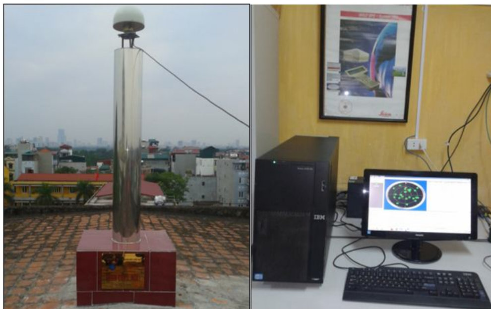
Figure 8. Installation of CORS N001 station system at Hanoi University of Mining and Geology.
